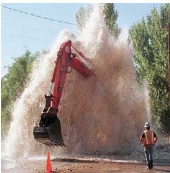
24" Water Main Hit
